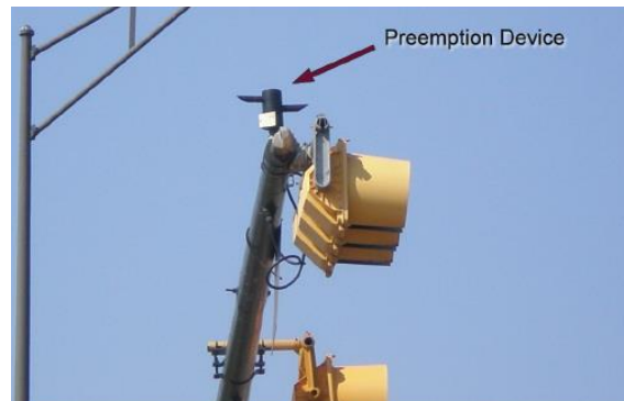
Traffic Signal Preemption (Texas)
