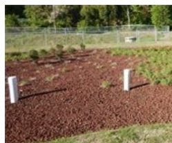
Bojangles' stormwater treatment train, designed by Kimley-Horn and Associates (2016 winners).
